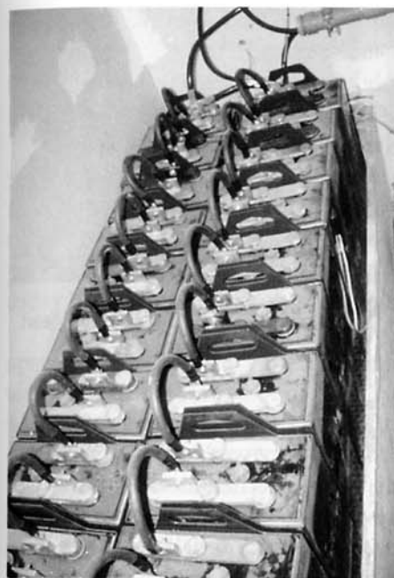
A bank of expensive, high-maintenance storage batteries are a necessary part of a solar power system.
