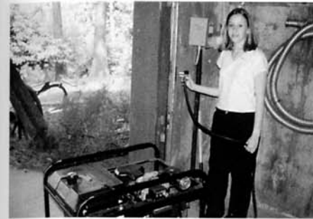
Many survivors who have reviewed their options have concluded they must use a generator.
