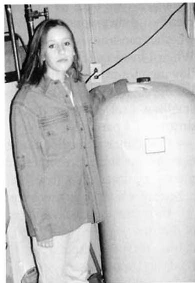
Controls and tanks for a do-it-yourself water system.
